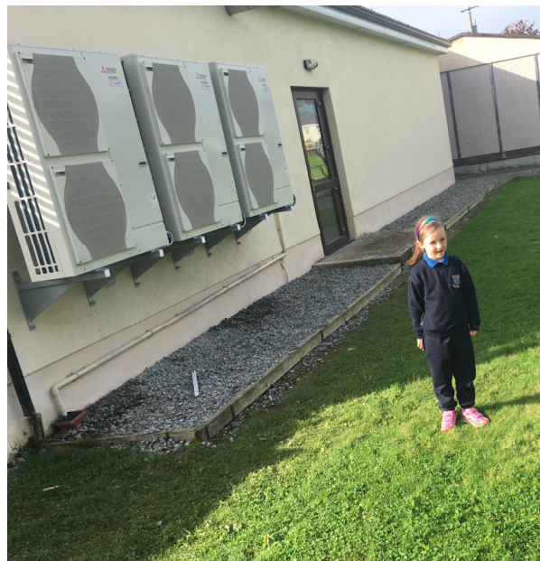
Figure 29 ASHP Units Installed at Youghalarra N.S.
