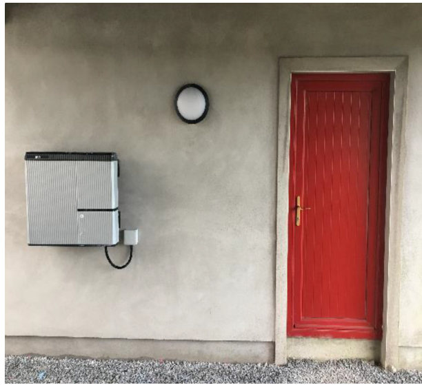
Figure 21 Battery Storage System installed at a Rural Domestic Dwelling
