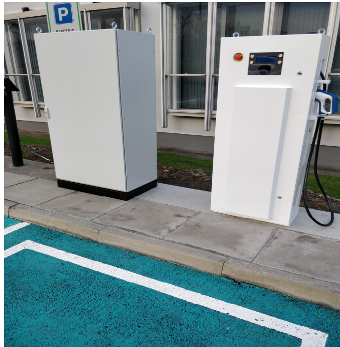
Figure 10 V2G Charger Infrastructure
