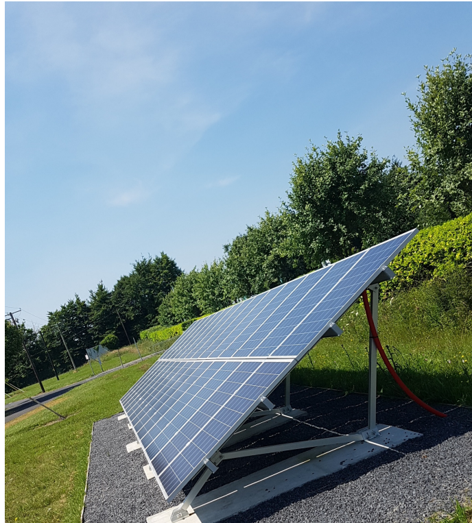
Figure 15 Solar PV Array in NTC, Portlaoise
